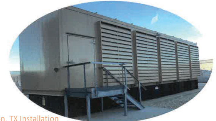
Houston, TX Installation
